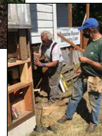
Charlie and volunteer John Goertzen make repairs to bay window structure in the front of the house, BCAC photo.
